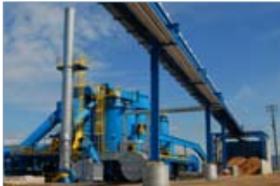
Tolko Biomass Gasification System
