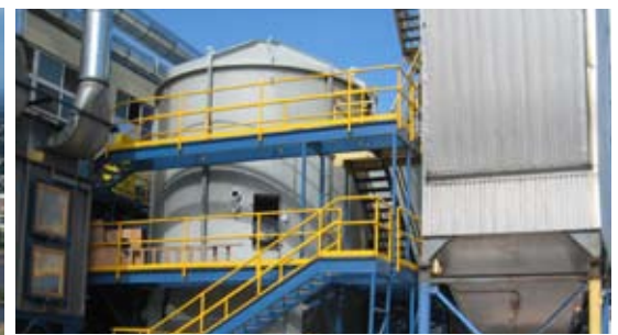
Kruger Biomass Gasification System
