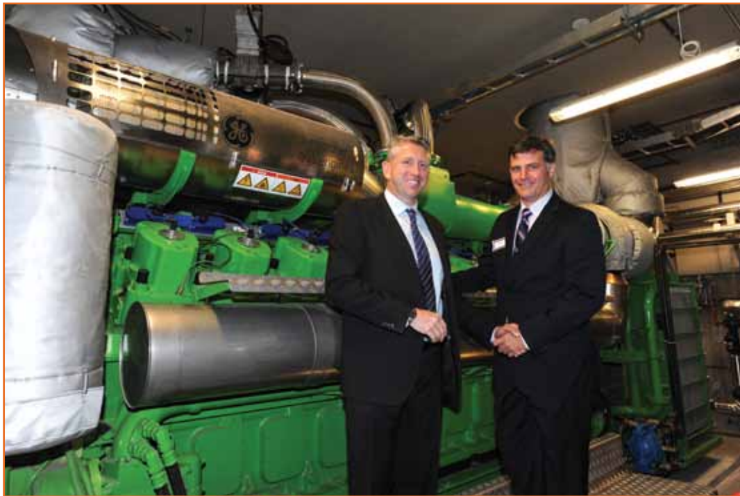
GE Canada Energy Financial Services MD Mark Tonner and Nexterra's Mike Scott in front of the Jenbacher engine
