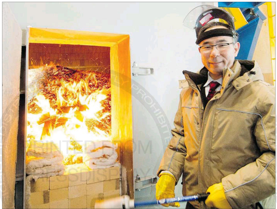
University of Northern British Columbia president George Iwama in front of the Nexterra biomass gasification system installed at UNBC. The plant's emissions were as good or better than natural gas, dealing with the thorny issue of air pollution from such plants.
