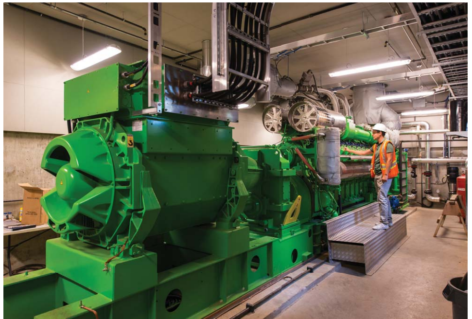
General Electric's Jenbacher engine at UBC uses syngas created by gasifying biomass to produce power and heat. Photos courtesy Nexterra Systems.
