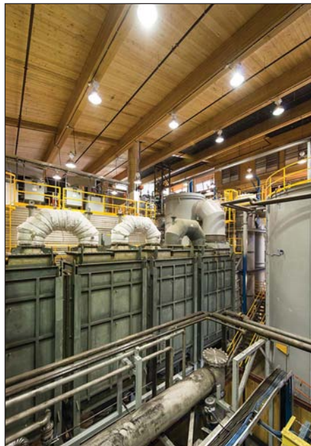
Nexterra's CHP system at UBC is the first energy-from-waste combined-heat-and-power system in the 2-10 MWe-size range in North America. Photos courtesy Nexterra Systems.
